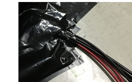
exit for signal cable
